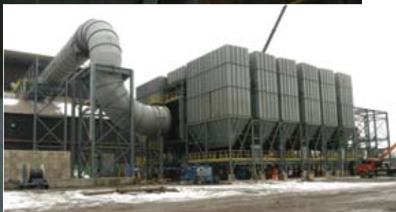
WCI Steel's new $29.3 million baghouse in Warren, Ohio, will reduce environmental emissions and support new federal air quality standards.
