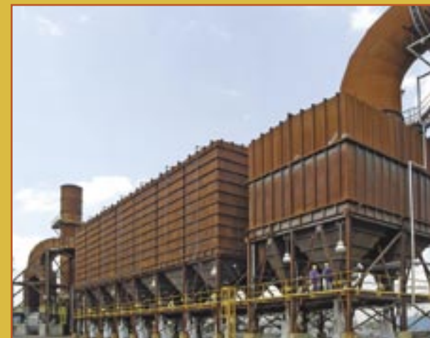
New blast furnace air emission controls at AK Steel Corp.'s Middletown facility capture fugitive air emissions.
