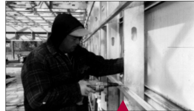
A builder demonstrates easy techniques of joinery for residential steel framing, which is increasingly popular among builders and consumers.
